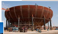
On-site fabrication pre-staging for construction: Unit 3 Containment Vessel Bottom Head and Ring 1
