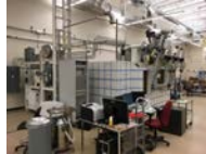
Electron Probe Micro-Analyzer (EPMA) installed in shielded enclosure
