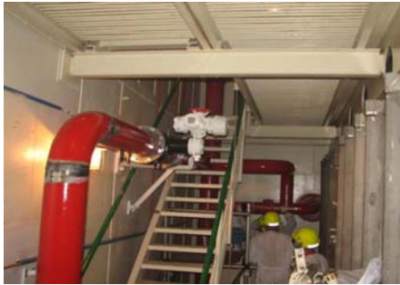
Containment vacuum breaker
