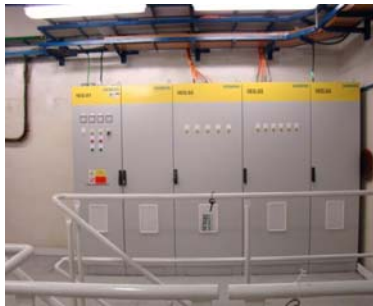
Alternative (seismically qualified) electric power system
