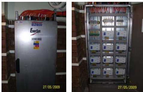
Battery monitoring system
