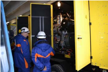
New mobile 0,4kV DG – 1/per unit
