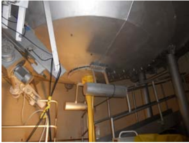
Bottom part of reactor shielding with floaters for outside cooling of RPV
