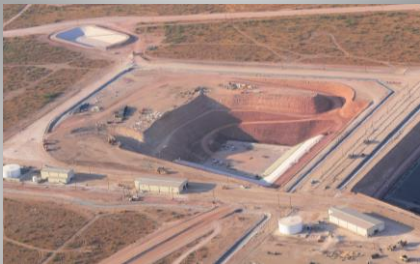
Aerial Photo Taken August 2011 by WCS Oblique photograph was taken looking to the southeast showing the Compact Waste Facility (center) and support facilities under construction
