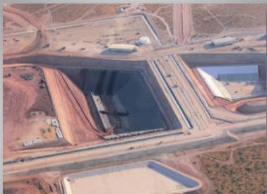
Aerial Photo Taken August 2011 by WCS Oblique photograph was taken looking to the north showing the Federal Waste Facility (center) & the Compact Waste Facility (right) & support facilities under construction
