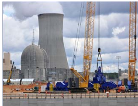
Plant Vogtle photo courtesy of Southern Company.
