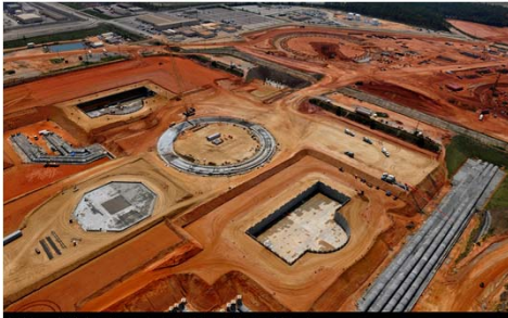
Aerial photograph of Vogtle 3 and 4 construction site. Unit 3 is located at left and top of photo and Unit 4 to the right and bottom. Heavy lift derrick crane foundation in center. August 11, 2011 © 2011 Southern Company, Inc. All rights reserved.
