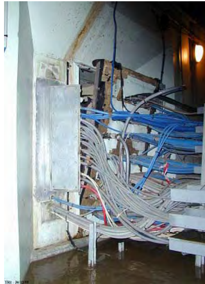
Failure of Cable opening
