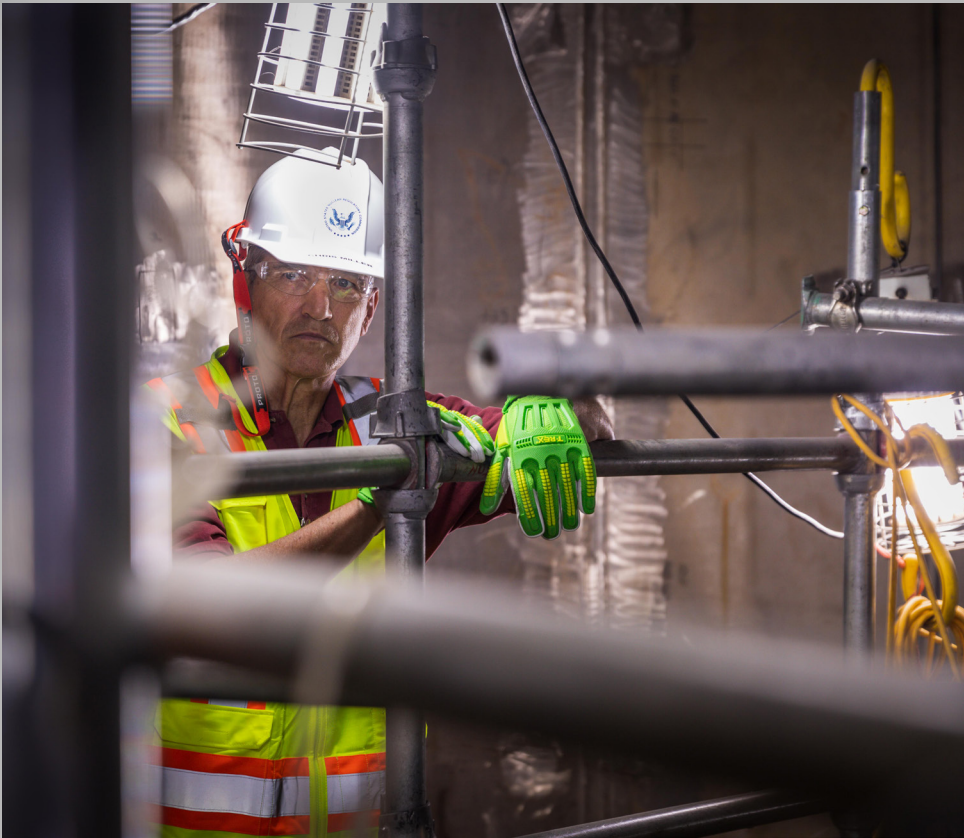
NRC Division Director Chris Miller observes new construction activities at Vogtle Units 3 and 4, in Georgia.
