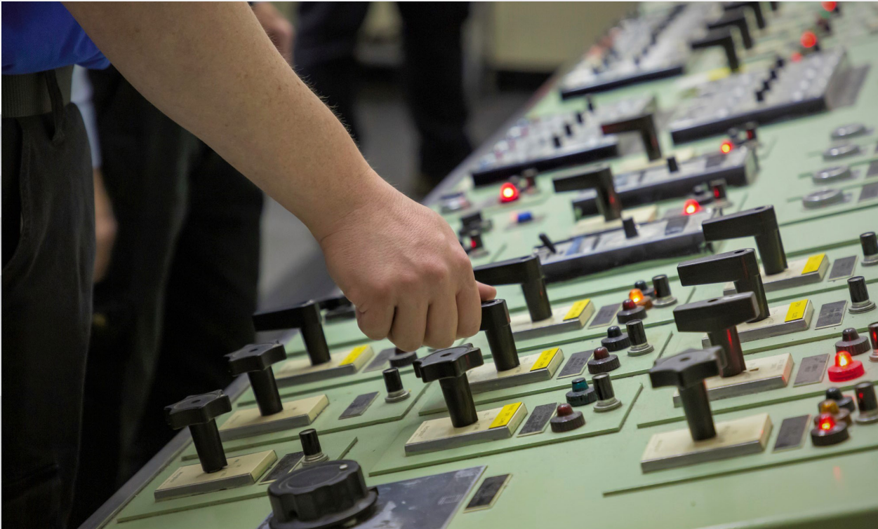
Indian Point nuclear power plant control room operators prepare for the final insertion of control rods in the Unit 3 reactor, part of the permanent shutdown of the site in New York. Not pictured NRC inspectors watching operations.
