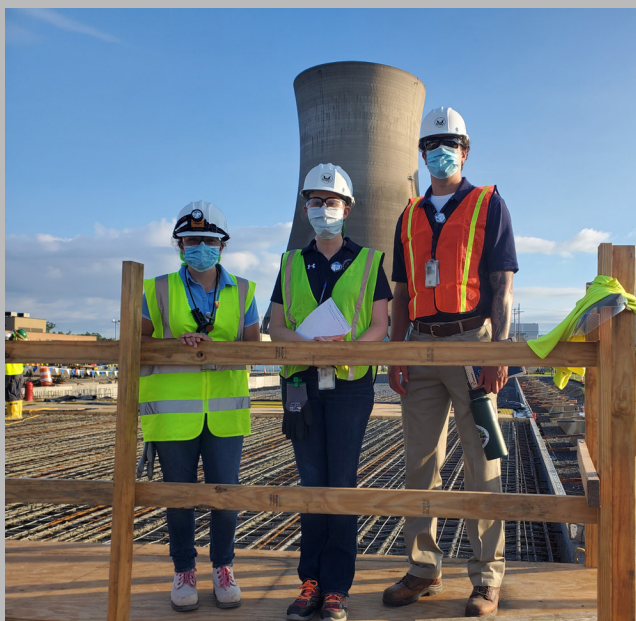
NRC inspectors (left to right) Katherine Warner, Liz Andrews and Mark Henrion observe workers preparing and pouring concrete for a dry cask storage pad on the Three Mile Island plant site in Pennsylvania.
