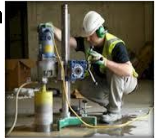
Concrete coring to obtain samples for evaluating effects of aging and environmental stressors.
