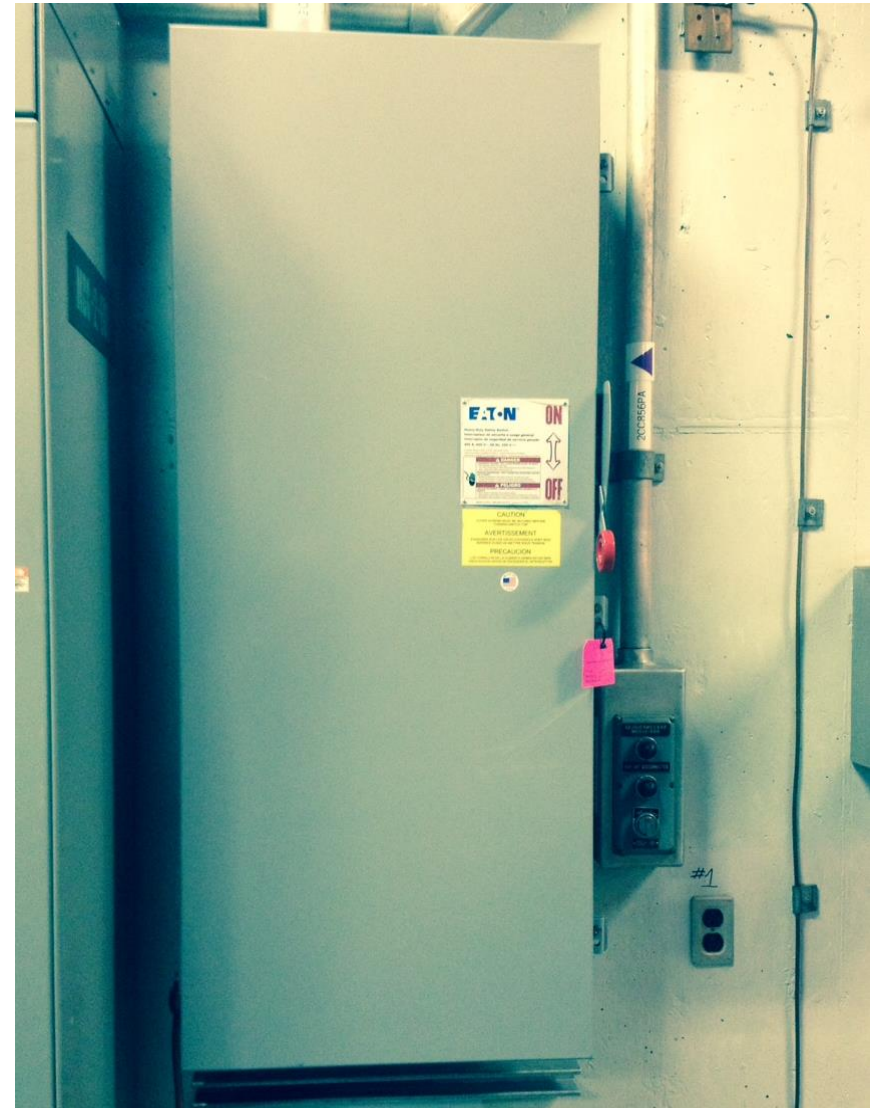
AC Power Quick Connection
