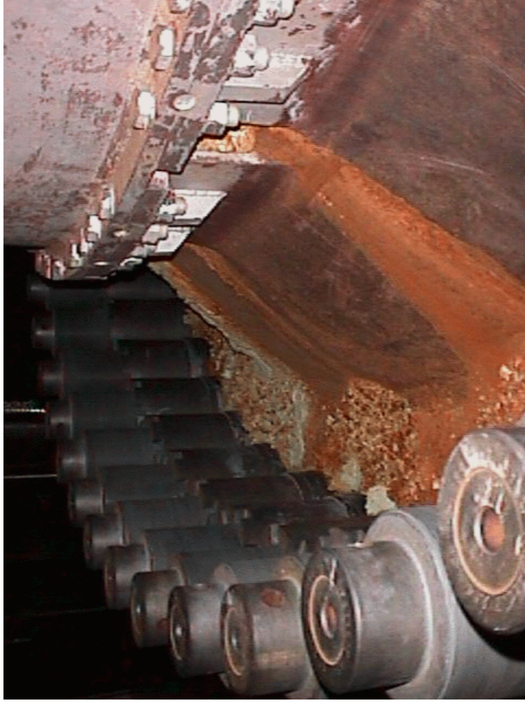
Figure 2-5 BORIC ACID DEPOSITS ON RPV HEAD FLANGE
