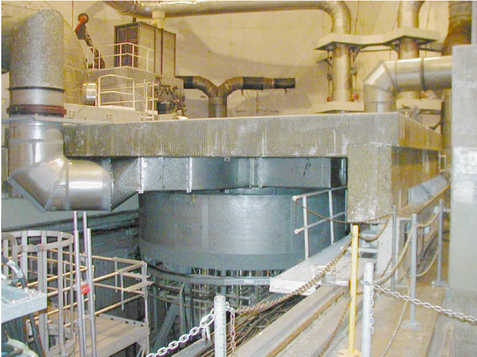
Attachment 2: Installed Missile Shield
