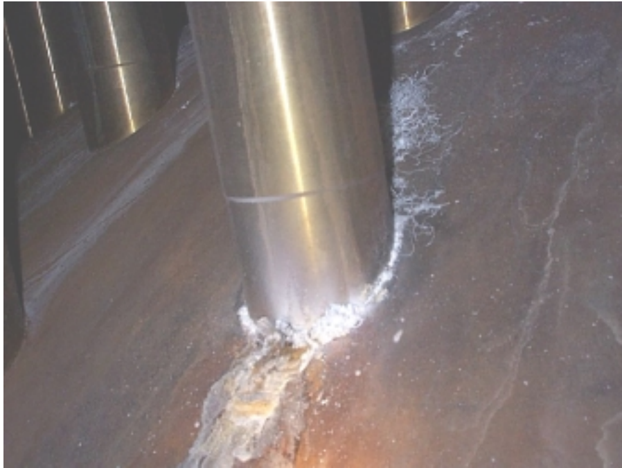
Figure 7 Visual Inspection of Oconee 3 Reactor Vessel Head (Leaking Nozzle 56)
