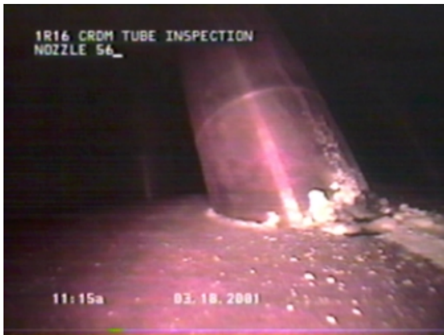
Figure 12 Visual (Video) Inspection of ANO-1 Reactor Vessel Head (Leaking Nozzle 56)
