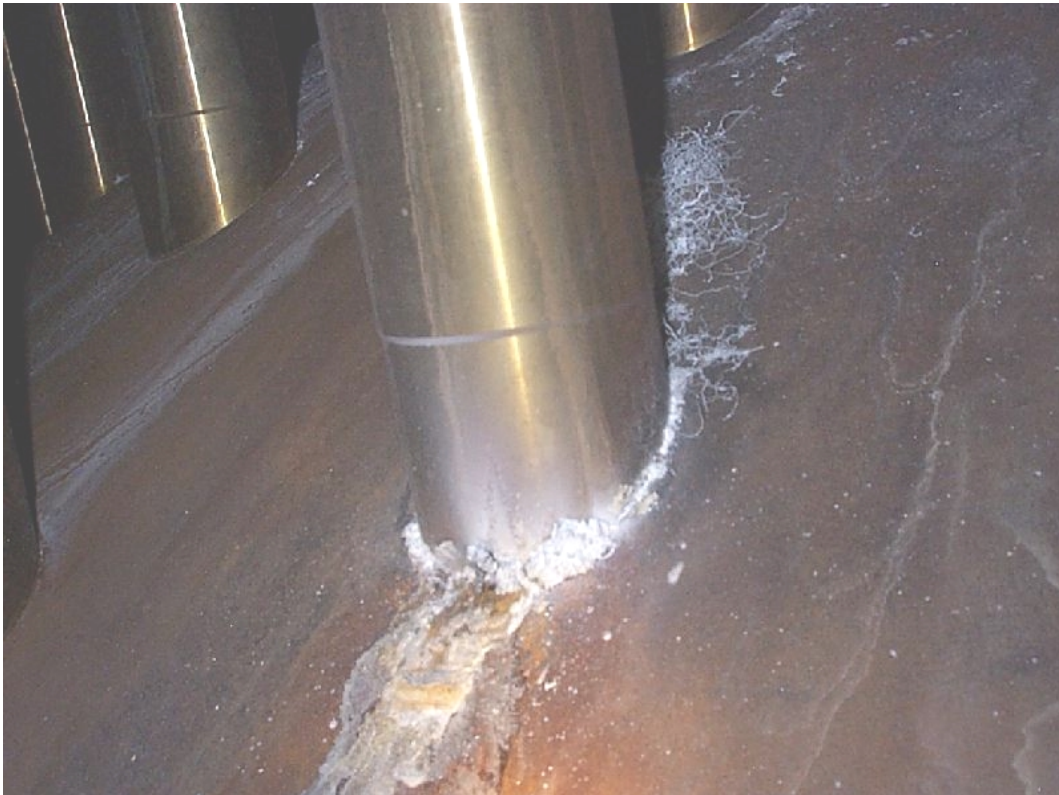
Figure 2-3 Leaking CRDM Nozzle at Oconee 3
