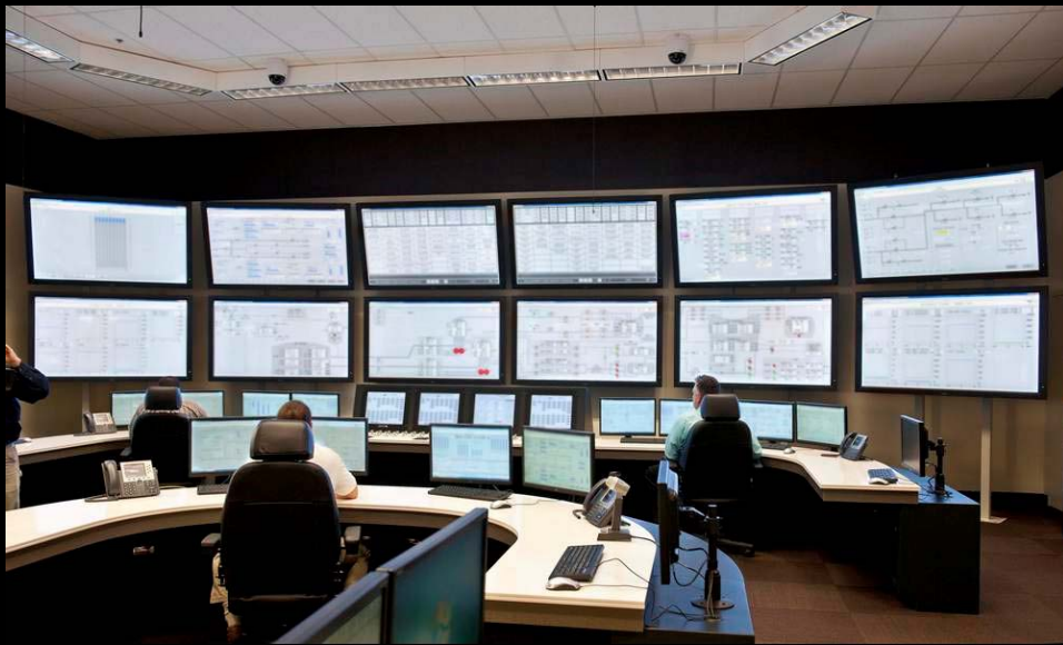
Testing of the Westinghouse AP1000 control room simulator software in preparation for training of Vogtle 3 and 4 plant operators.
