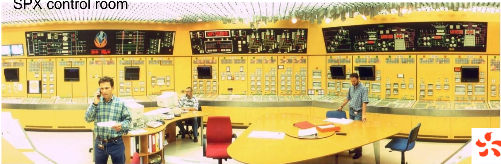
SPX control room
