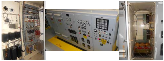
EDG (emergency diesel generator) Excitation Systems
