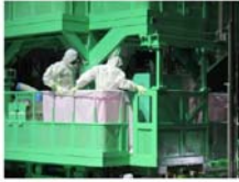
The NRA Safety Inspectors watch TEPCO's spent fuel removal operation on the fuel handling machine.
