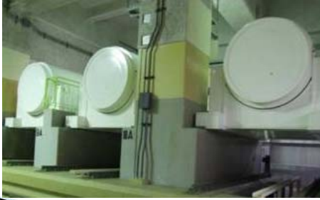
• Dry metal storage casks for spent fuel at Fukushima-1 NPP
