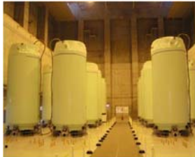
Storage casks at Tokai-2 NPP
