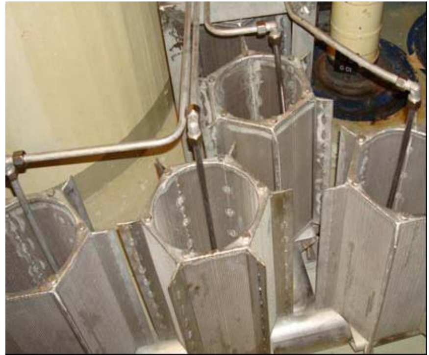
Loviisa NPP upgraded sump strainers and back flushing system (1993)
