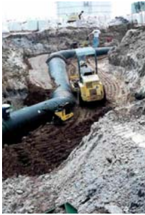
Buried HDPE Pipe
