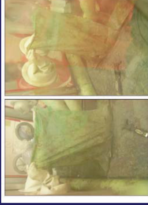
Figure 5. Removal of cured Decon Gel 1101 as a strippable film from cast steel glove-box floor.
