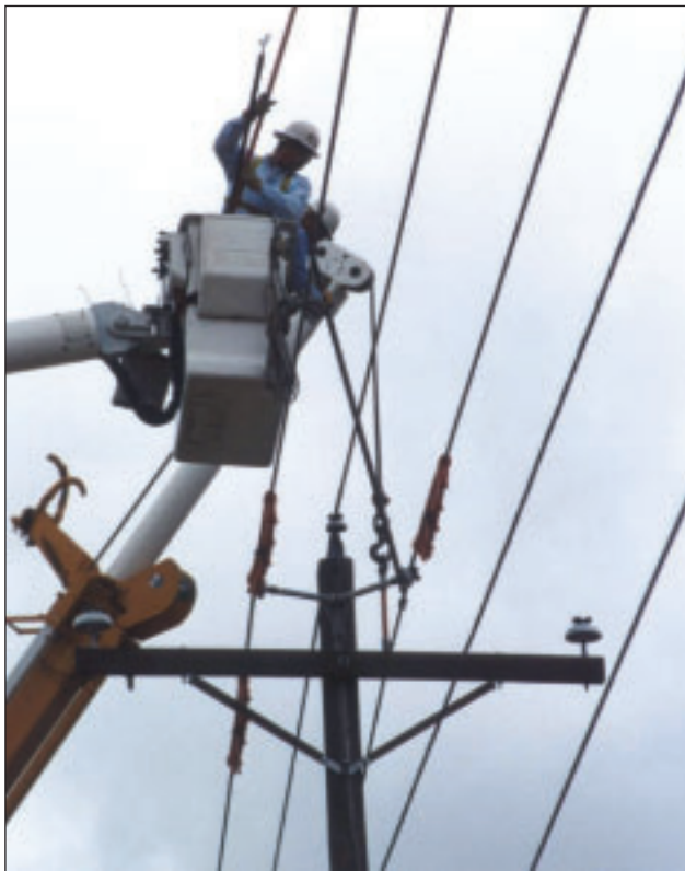
FIGURE 7.2: Reframing a crossarm to prevent avian electrocutions.
