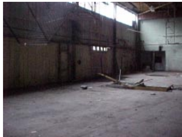
Figure 8 - Area of Building Where Sign Was Damaged
