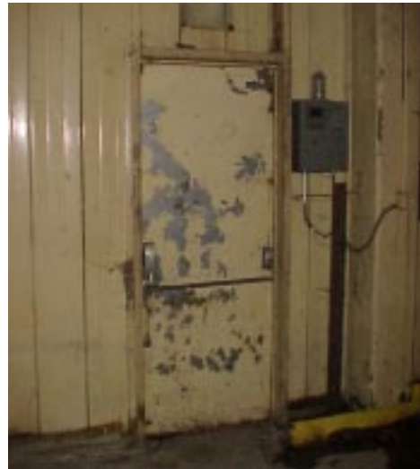
Figure 6 - Door where Broken Sign was Installed
