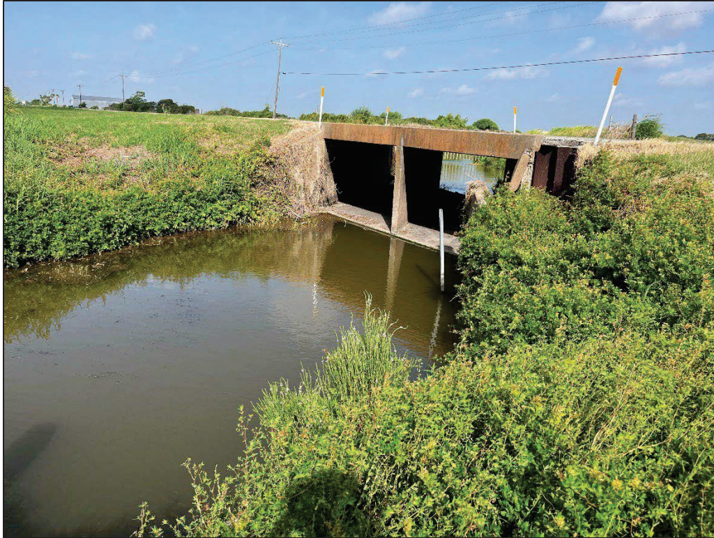
Figure 5-11. Offsite surface water monitoring (WCC-3); facing southeast.
