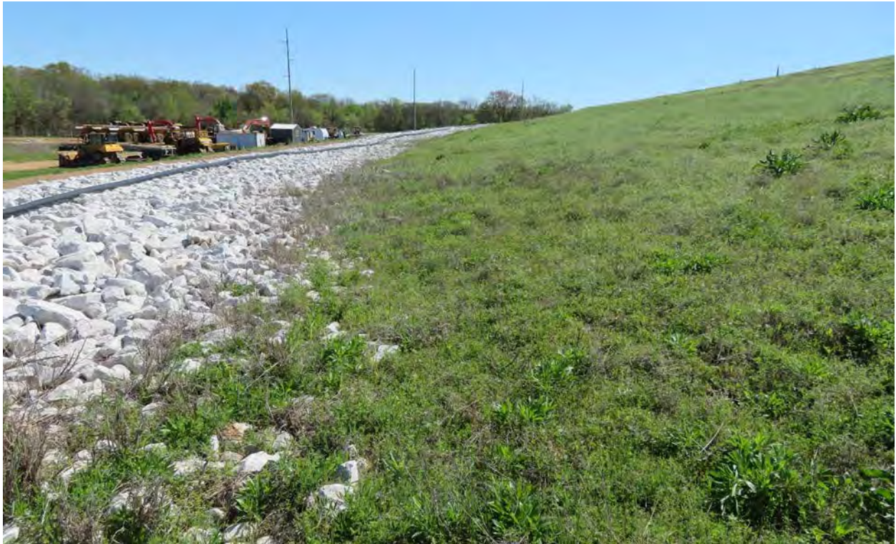
Photo 20. North side of Cell showing apron bench and vegetated slope, looking east (Apr 2024)
