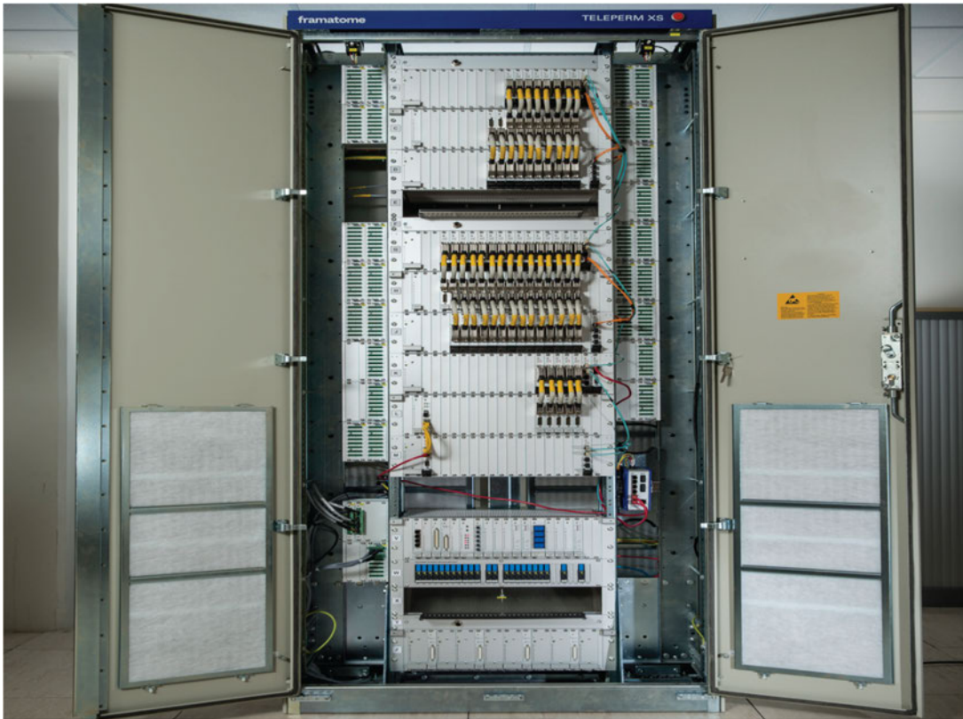
Figure 1: TELEPERM XS Compact in Cabinet 3
