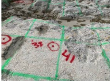
DM #5 Auxiliary Bldg (At the 41 marked location)
