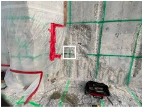
DM #8 Auxiliary Bldg (Lower wall location marked by white box in photo)
