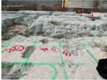
DM #5 Auxiliary Bldg (At the 41 marked location)
