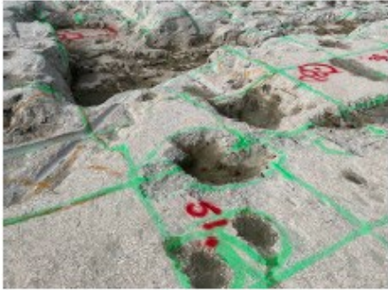
DM #3 Auxiliary Bldg (At the 51 marked location)
