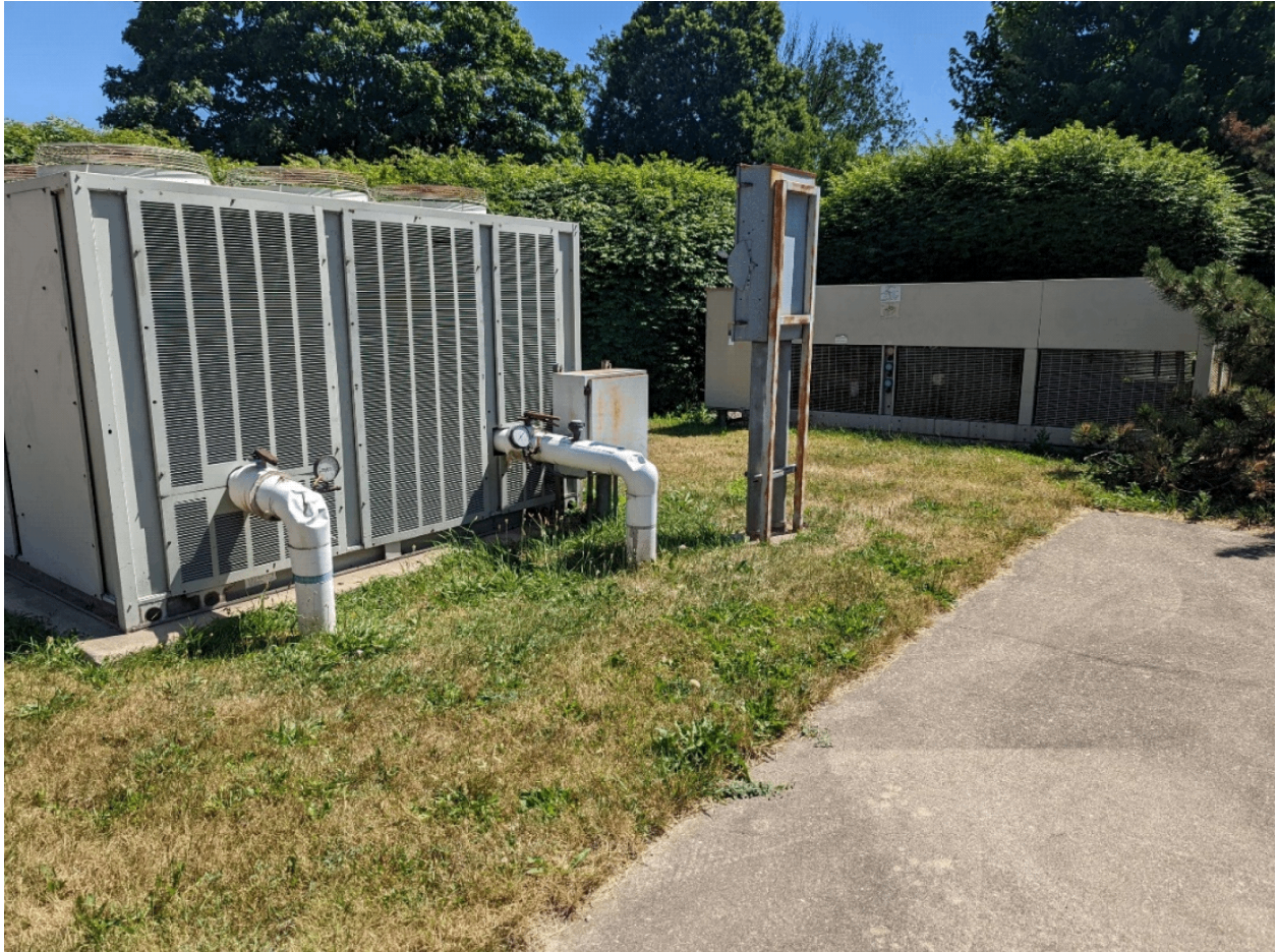
Figure 4-7 GSL Mechanical Equipment Located East of The GSL
