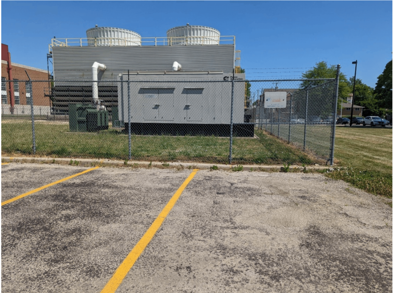
Figure 4-6 North View of Abbott Cooling Towers From The Site
