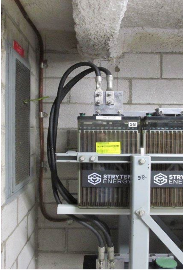
Figure 5. Unsupported Inter-Tier Cabling
