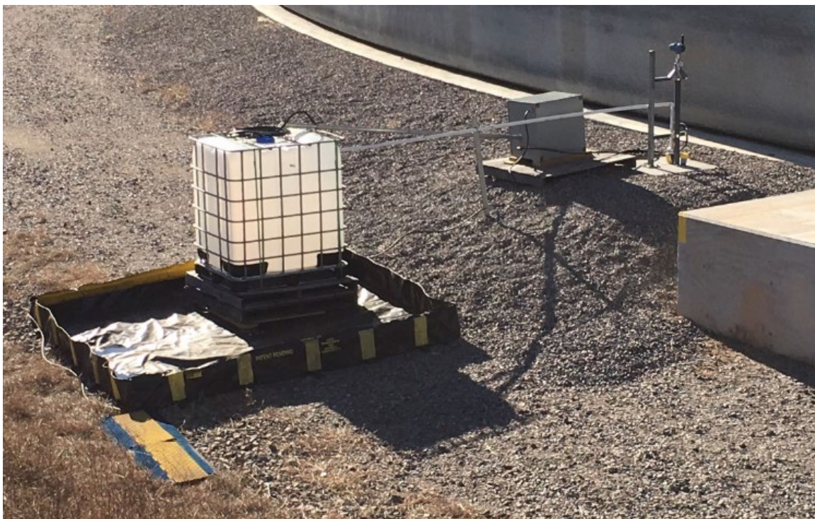
Figure 3.2-1: SSF-TMC-18-003, De-Watering Pump at the East Sump of SDU 6
