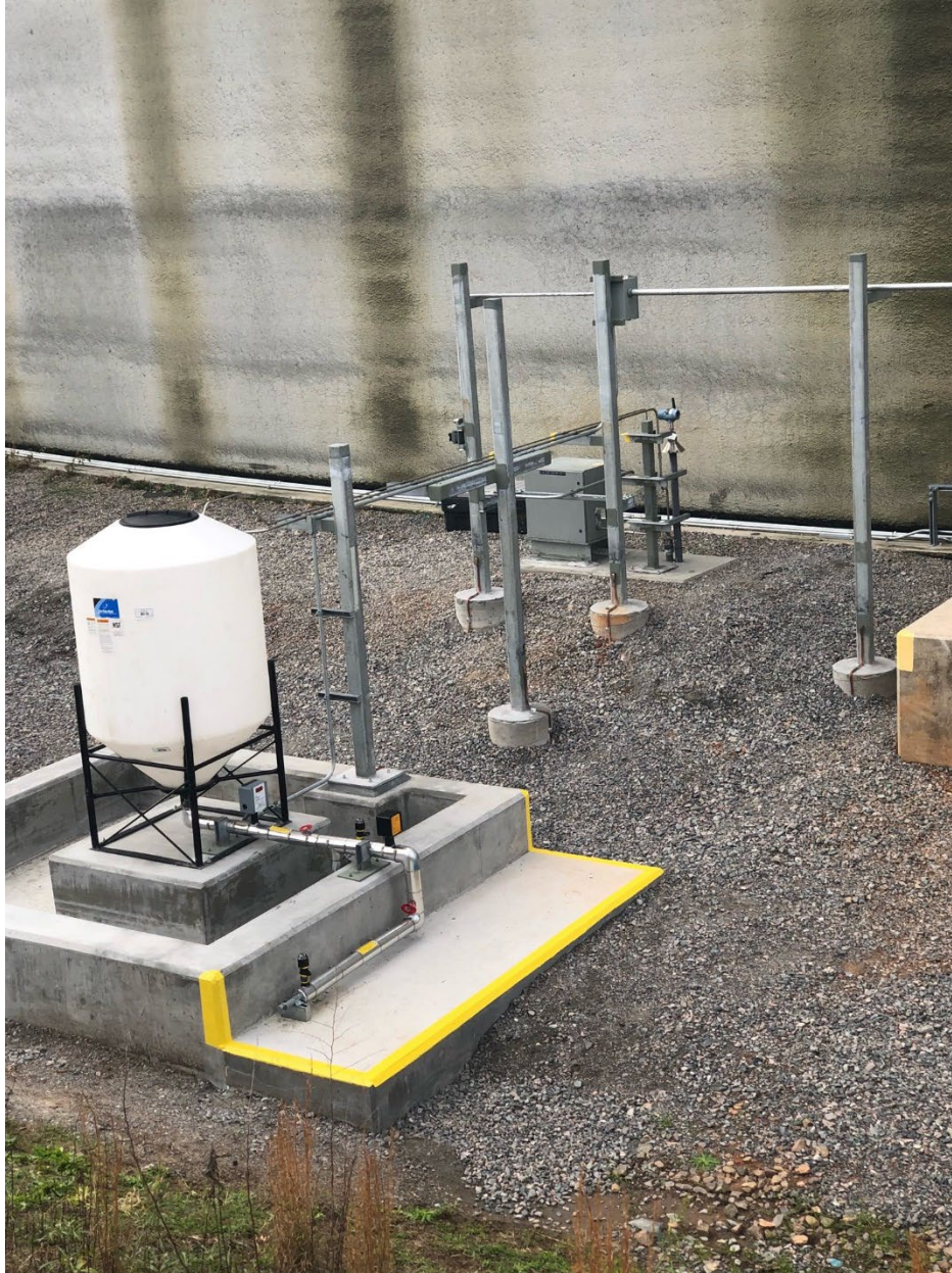
Figure 3.2-2: M-DCP-Z-20001 De-Watering Pump at the East Sump of SDU 6
