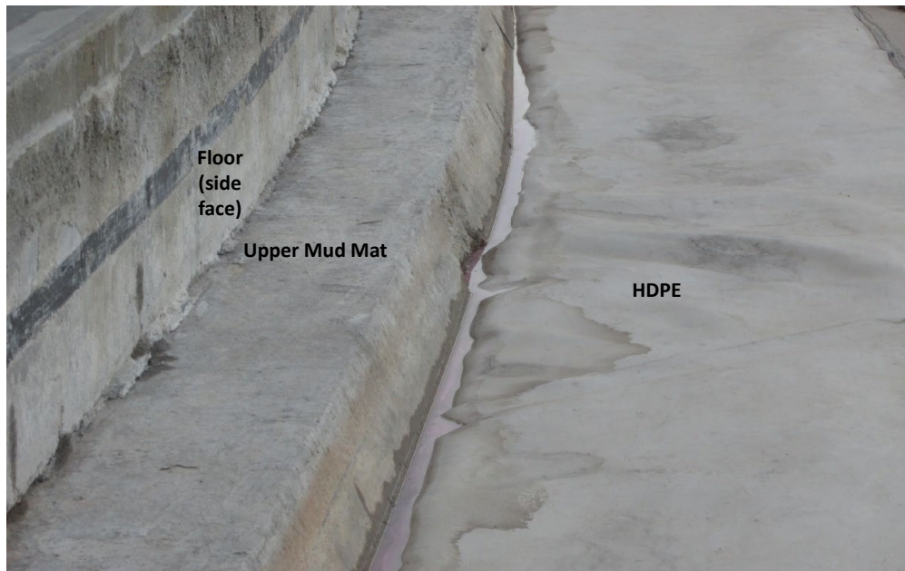
Figure 2.3-6: Observed Leak from First Leak Tightness Test of SDU 6, November 2015 (6 of 6)
