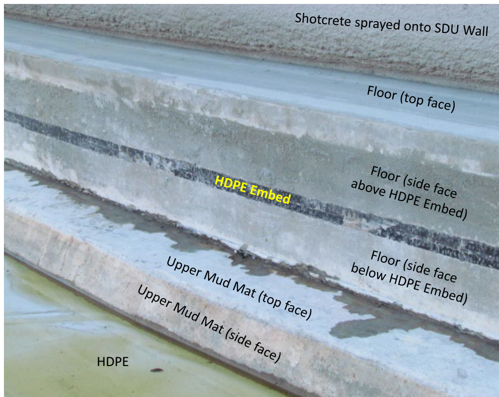
Figure 2.3-1: Observed Leak from First Leak Tightness Test of SDU 6, November 2015 (1 of 6)
