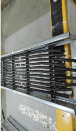
Typical configuration of uncoated cables attached to a tray.
