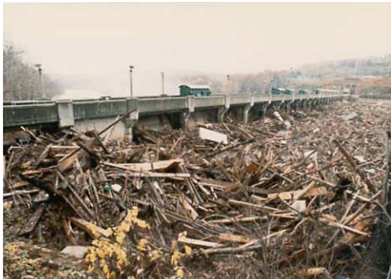
Figure 9. Debris Upstream of Lake Lynn Dam after 1985 Flood Event (Schadinger et al., 2012)
