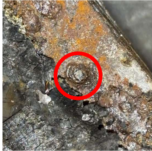
Short Circuit Path – Photo 2
