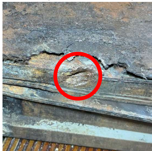
Short Circuit Path – Photo 6
