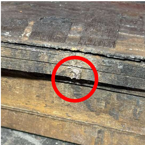
Short Circuit Path – Photo 3
