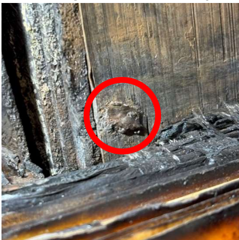
Short Circuit Path – Photo 5
