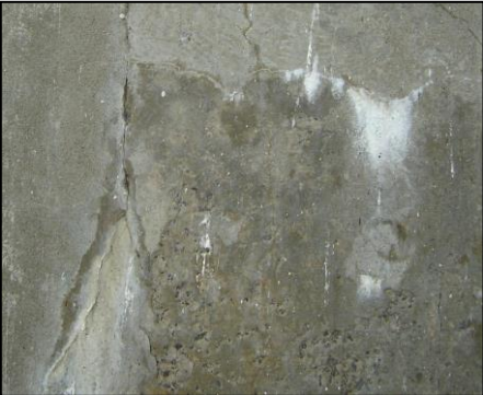
Concrete Wall Alkali Silica Reaction
