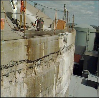
Fill Concrete Degradation
