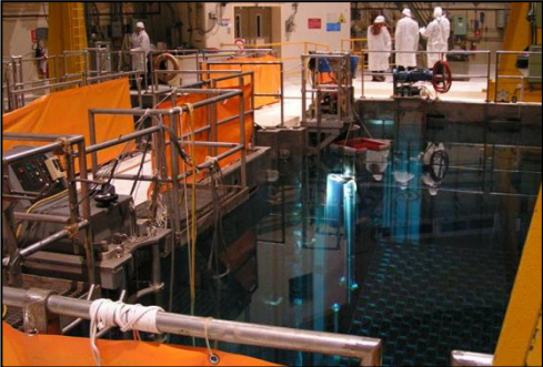
Spent Fuel Pool Leakage
