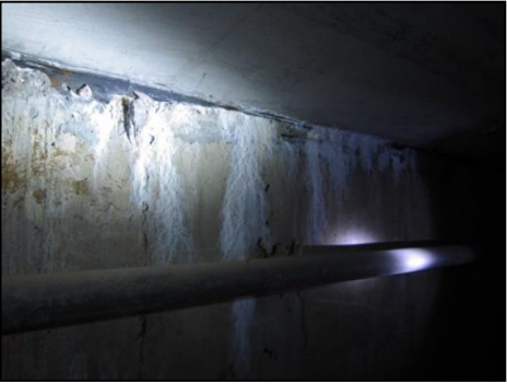
Underground Structure Leaching and Efflorescence
