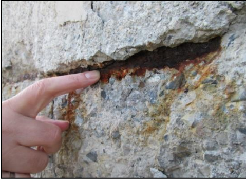
Reinforcing Steel Corrosion
