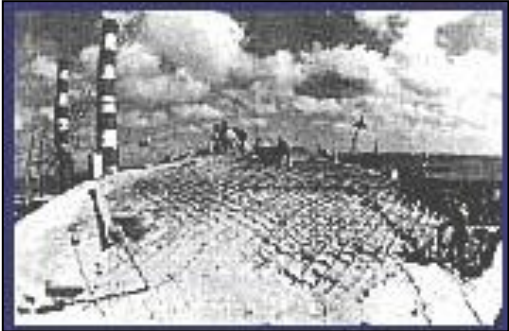
Containment Dome Delamination
