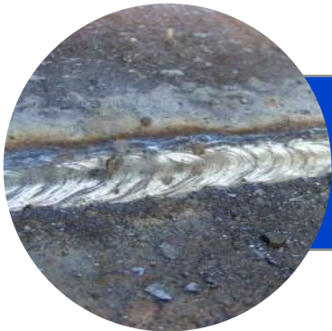
Latent Weld Defect
