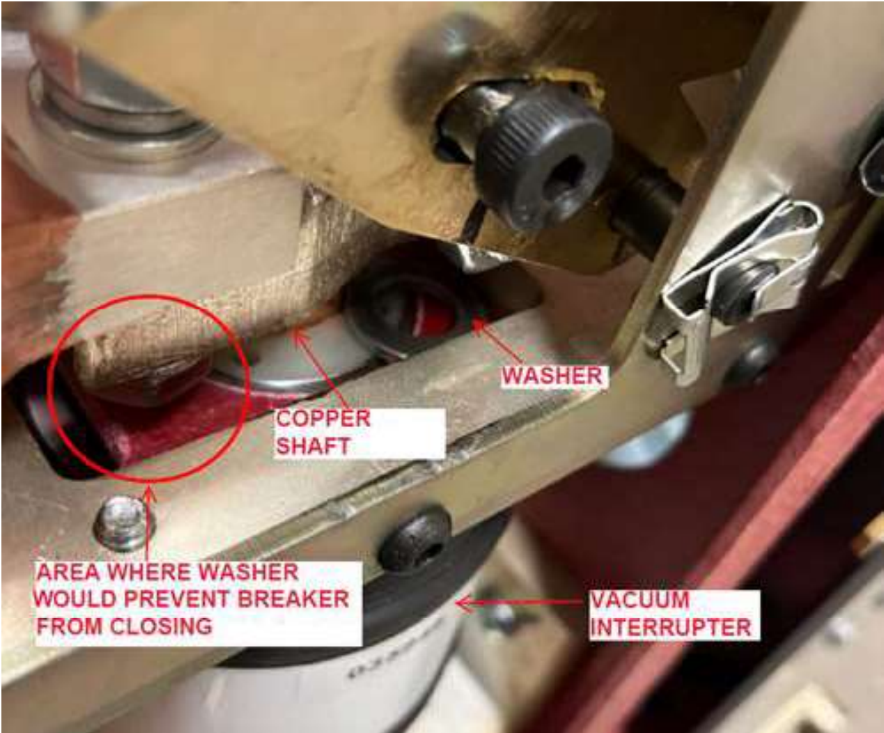
Figure 1 - Image of Breaker with Unrestrained Washer
