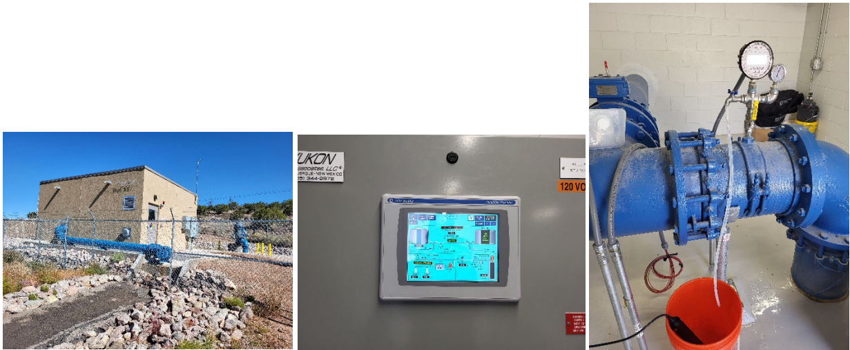
Photographs 2a, 2b, 2c – BSAG-12 sample location. Municipal supply well.
