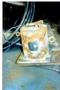
GAUGE PAINTED OVER
