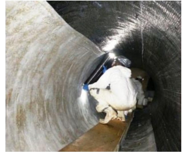
Photo Credit: Dominion Energy & Structural Technologies, 2018 EPRI Summer BPIG Meeting
