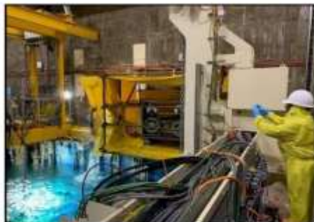
Observing decommissioning activity at San Onofre Nuclear Generating Station, San Clemente, California (Source: nrc.gov)
