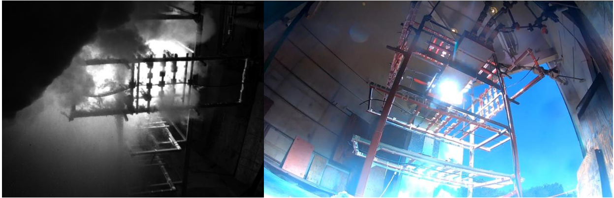
Figure 3-25: From left to right: Phantom v7, 4,000 fps, at top northeast side; GoPro at floor at north side with view of the first frame of the arcing 2.4 seconds from trigger.
