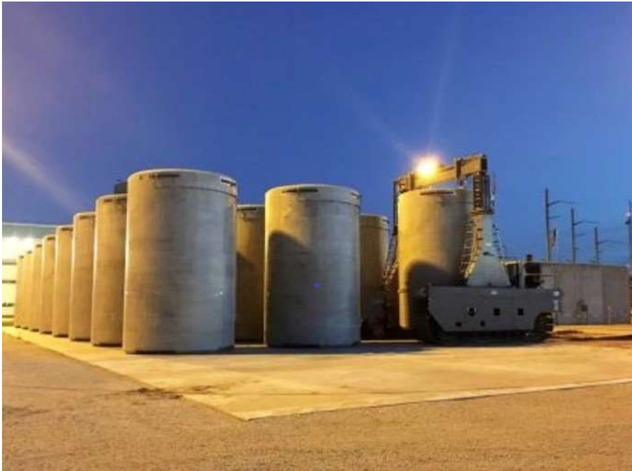
Spent Fuel Dry Cask Storage
