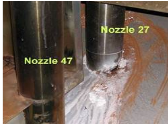
Leaking PWR CRDM Head Penetrations
