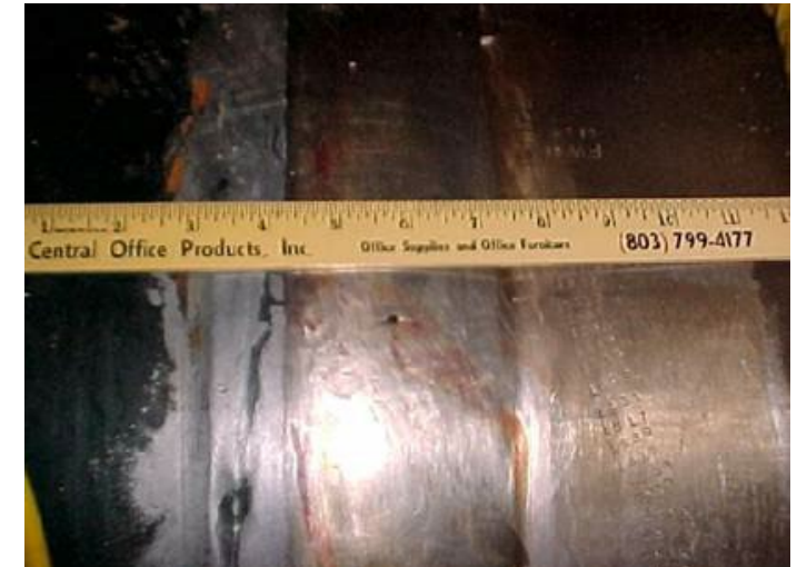
V.C. Summer Crack in RCS hot leg nozzle to pipe weld (Fall 2000)
