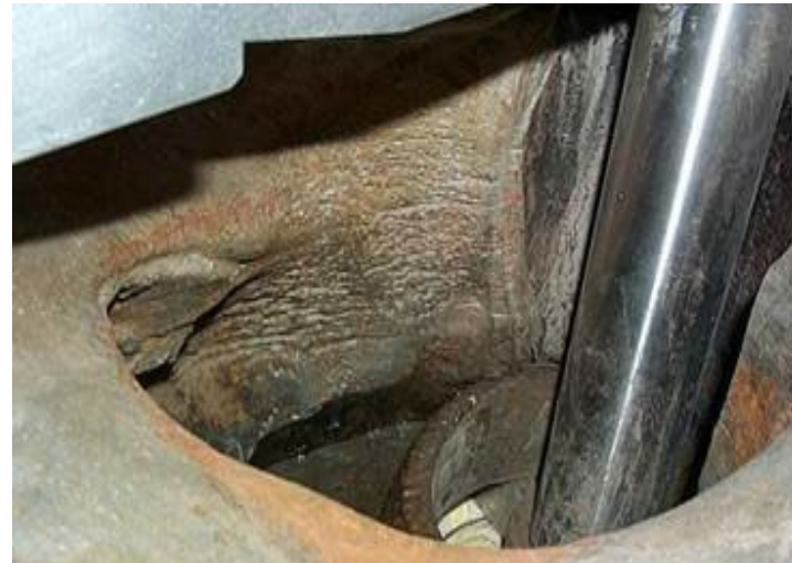
Davis – Besse CRDM penetration leakage/head wastage (March 2002)
