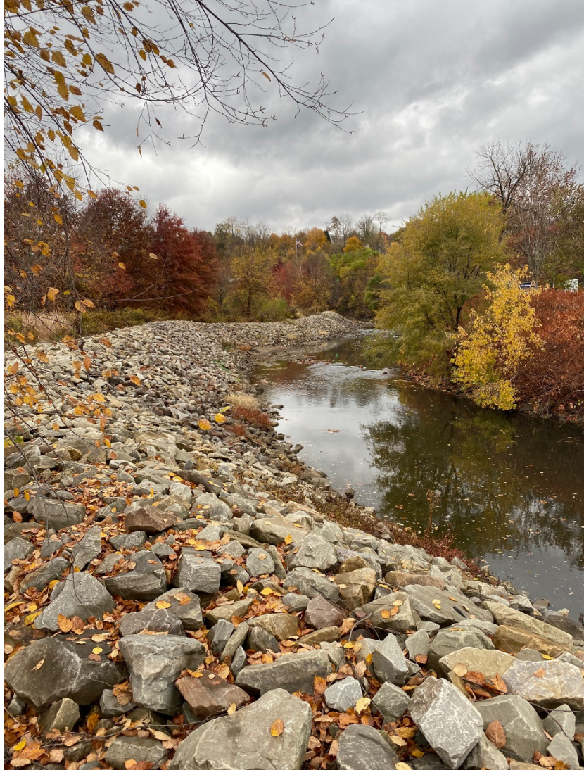
Fig. 1: Canonsburg site – Riprap stabilization between site boundary fence and Chartiers Creek (looking north to northwest); image captured on October 26, 2022.
