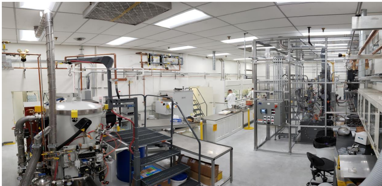
The TRISO-X Pilot Facility operates inside Oak Ridge National Laboratory via a public-private partnership and produces kilogram quantities of HALEU fuel.
