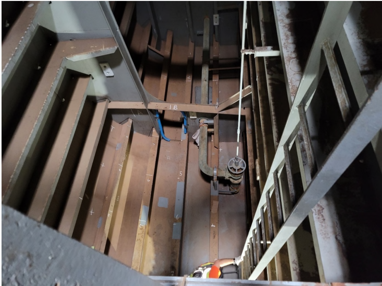
Photograph 2-1 Tank 9P Access Ladder, Cutout Valve, and Tank Bottom
