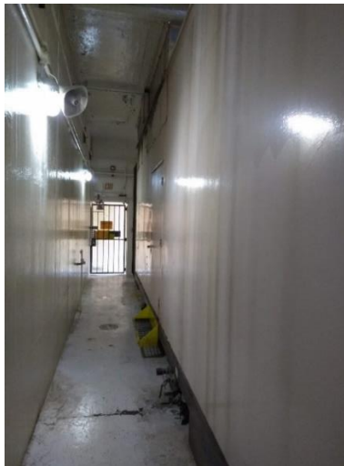
Figure 5-3 Hallway in the EDG Room (Courtesy of Oyster Creek NPP)
