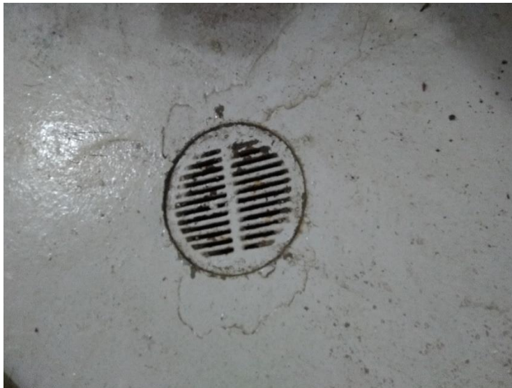
Figure 5-5 Floor Drain in the EDG Enclosure (Courtesy of Oyster Creek NPP)
