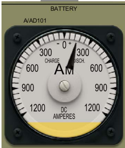
AMMETER SELECTOR SWITCH in POSITION 1
