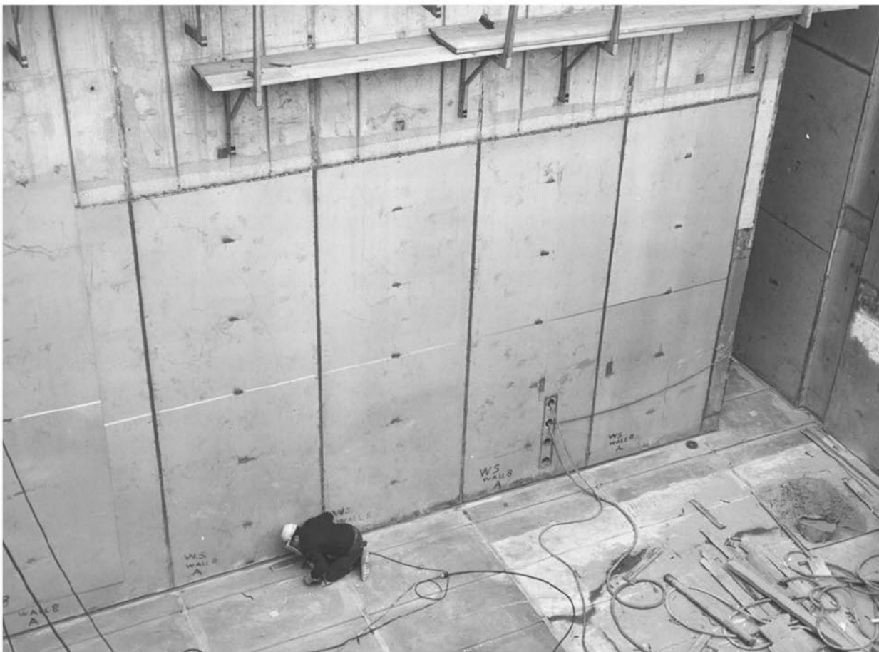
Figure 5-12. Stainless Steel Basin Liner. Both storage basins and the unloading basin are completely lined with stainless steel sheets (304L) placed flush against the concrete walls and floor, welded to a grid of stainless steel embedments.
